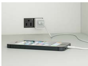
Interior Power Outlet
